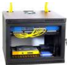
Server & Network Rack
